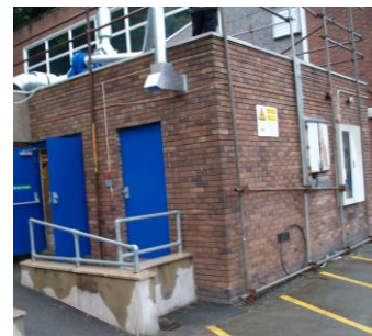
External bulk Chemical Store
